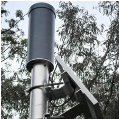
Dipstick Flood Alert System Figure 42.
